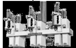
Automated Switched Cap Banks
