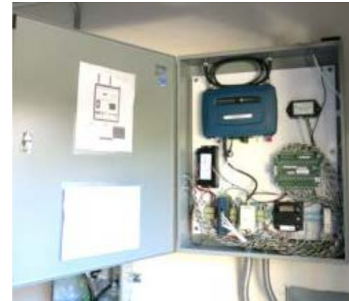
Home Data Monitoring System
